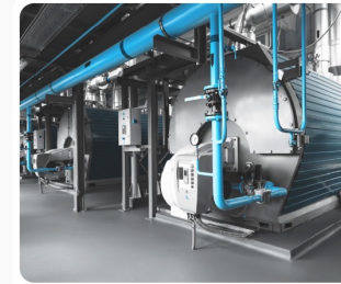
Heating & cooling systems
