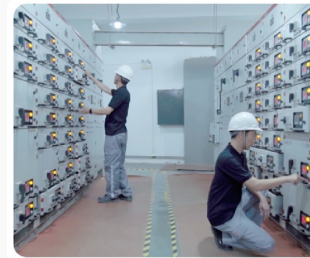
Electrical & high-voltage (HV)
