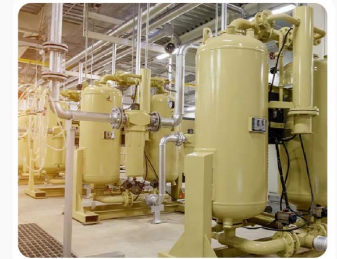
Compressed air, mechanical & hydraulics
