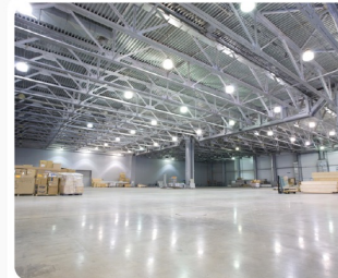
Lighting & earthing systems
